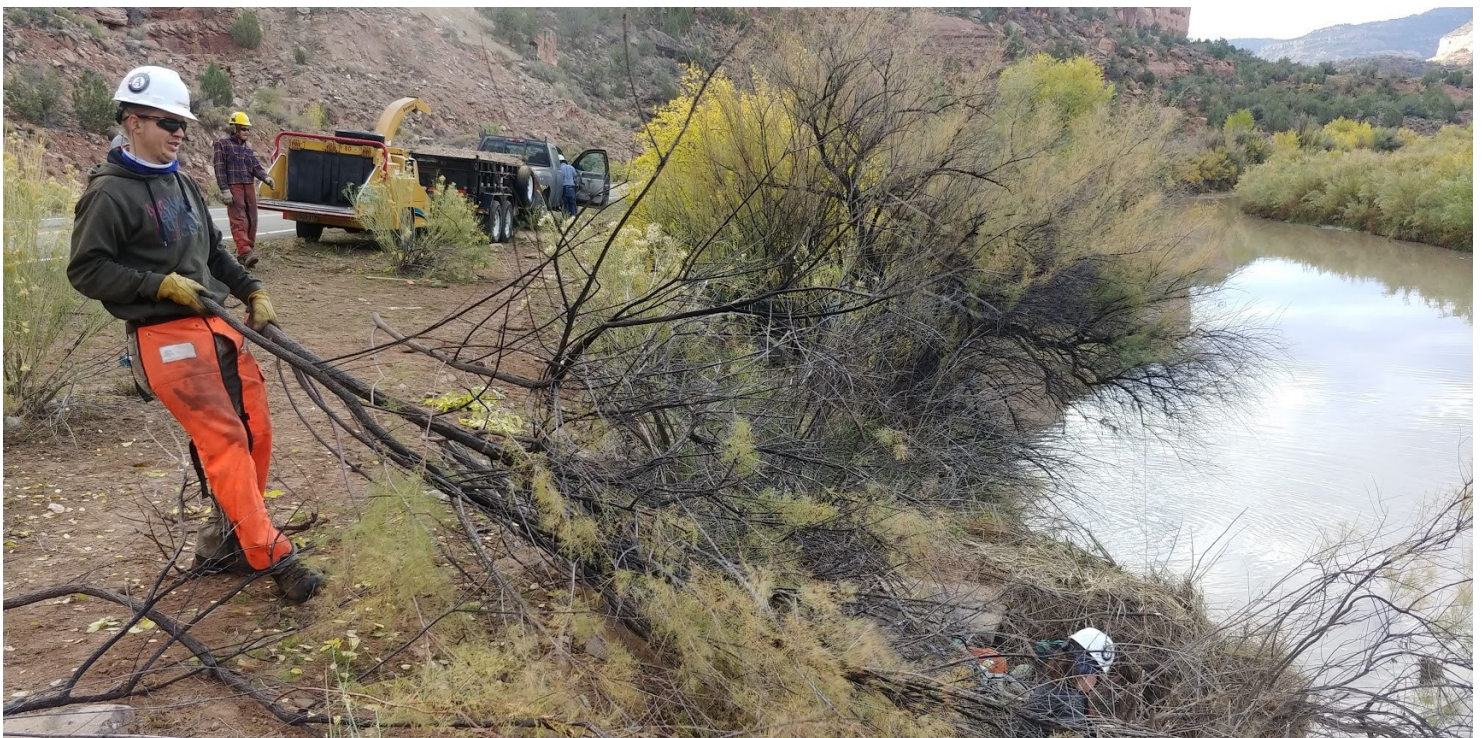
Saw crews from Western Colorado Conservation Corps remove tamarisk and drag cut limbs to a chipper along a narrow bank between Hwy 141 and the river, improving visibility and safety along the windy road
