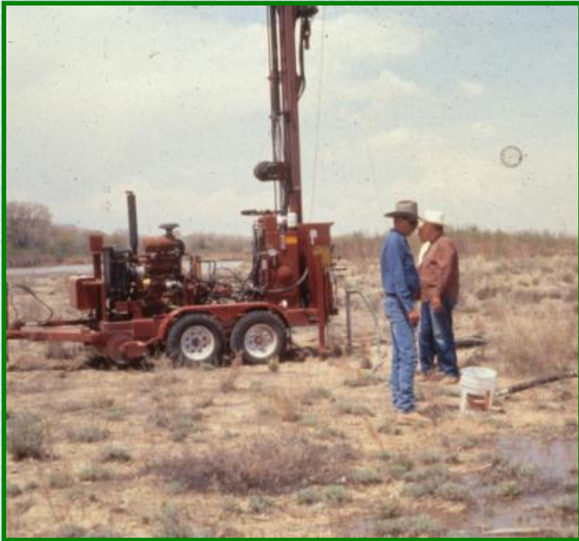
Drilling a shallow well on the west side of the Rio Grande in Albuquerque, New Mexico.
