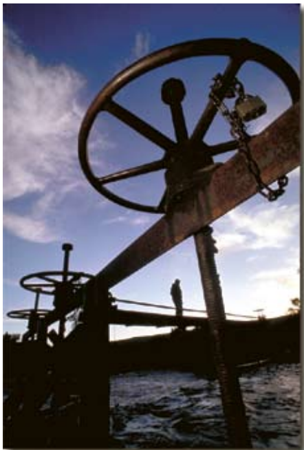
An irrigation headgate near Kremmling, Colorado controls the amount of water diverted from the Colorado River.
