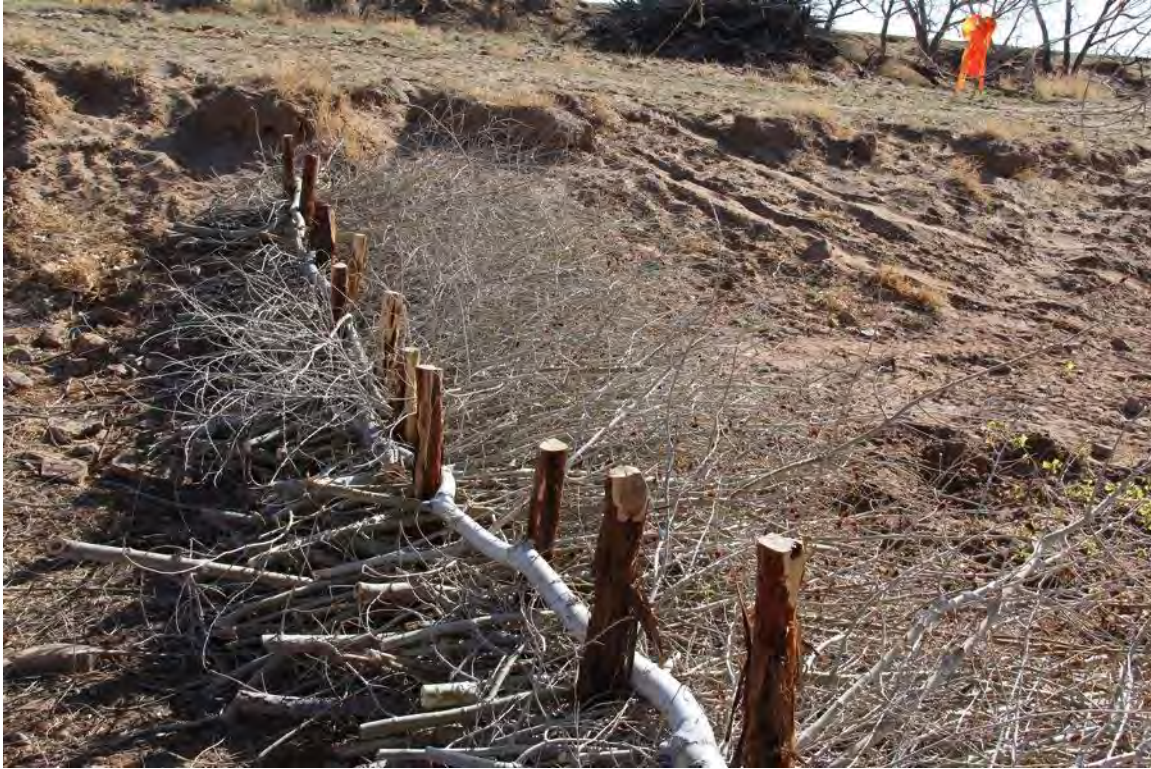
Figure 82: BDA interwoven with cottonwood branches parallel and perpendicular to the stream flow. The perpendicular, downstream (left to right) branches are placed to limit the development of a downstream scour pool during high-flow events, which could compromise the integrity of the structure. Photo courtesy of Seventh-Generation Institute.
