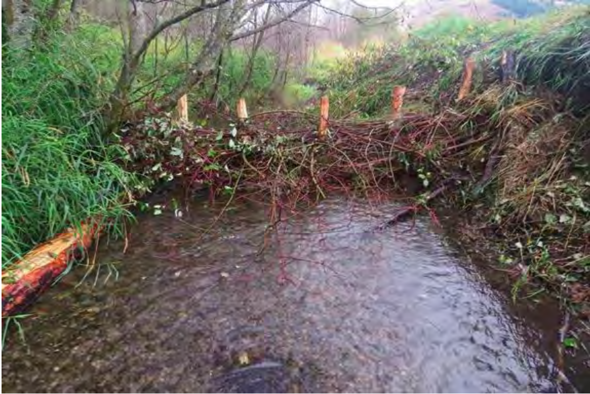
Figure 75: Pilings woven with live red oiser dogwood, some of which was planted directly into the exposed bank to facilitate resprouting
