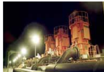
Yuma Desalting Plant, photo credit: Bureau of Reclamation
