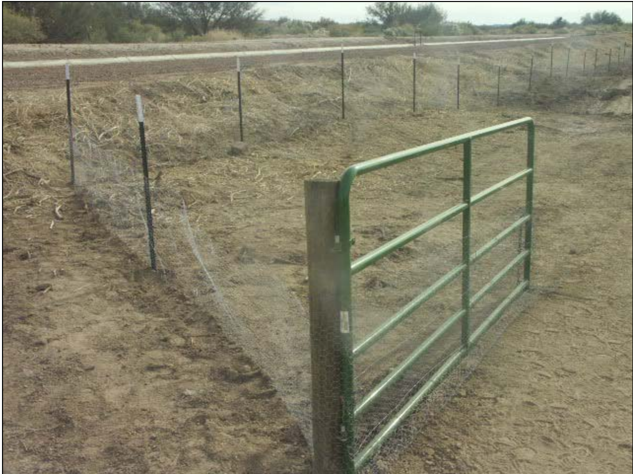
Figure 14. Rabbit-proof fencing with access gate installed around the perimeter of Demonstration Studies 1 and 2A, Cibola National Wildlife Refuge, Cibola, Arizona. The fencing was successful in excluding rabbits from study sites, but was also successful at retaining rabbits within that were trapped by the fencing installation – particularly for Study 1.
