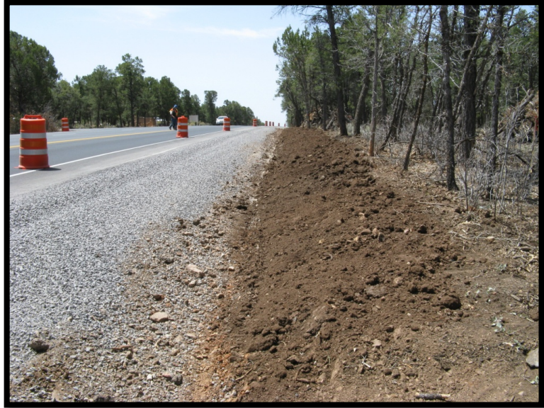
Topsoil that was properly dried and applied at the appropriate depth. This soil is well scarified and ready for seed and mulch treatment.
