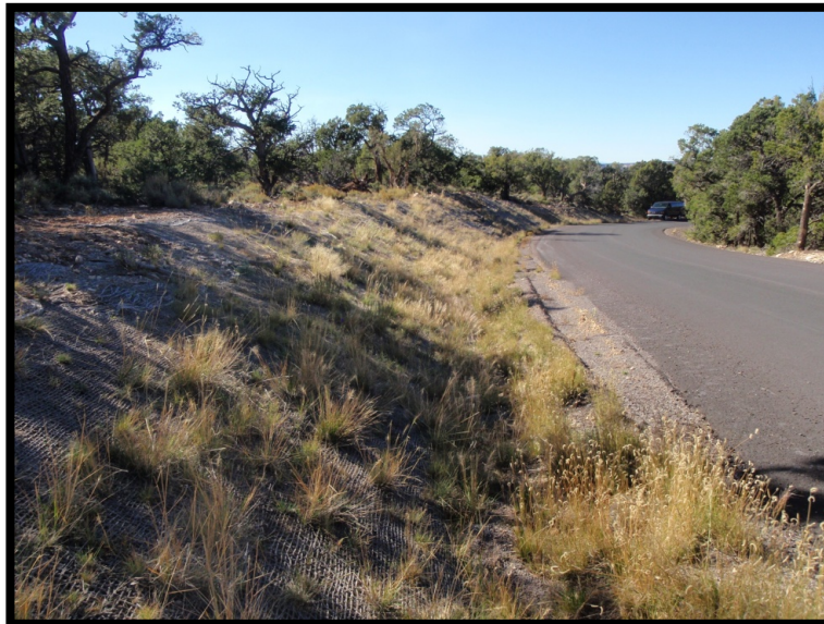
The same 3:1 and greater slope three years after seed, hydromulch, and blanket treatments. Note the healthy and robust establishment of native vegetation that ultimately stabilized the slope.
