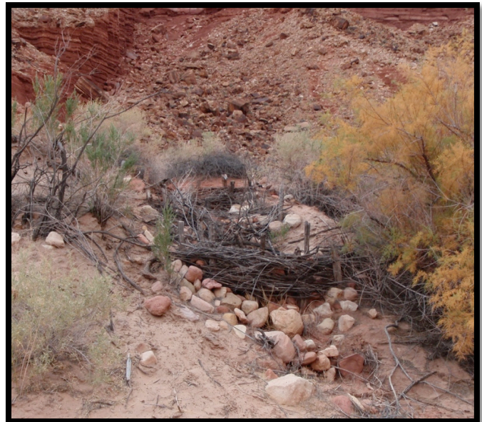
Zuni check dam installed at Soap Creek Camp., along the Colorado River.
