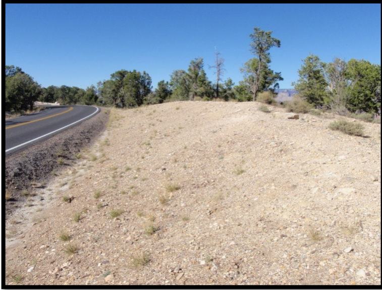
A 3:1 slope with seed and hydromulch treatment only, three years after seeding treatment. Note the very sparse vegetation establishment on a slope of this grade.
