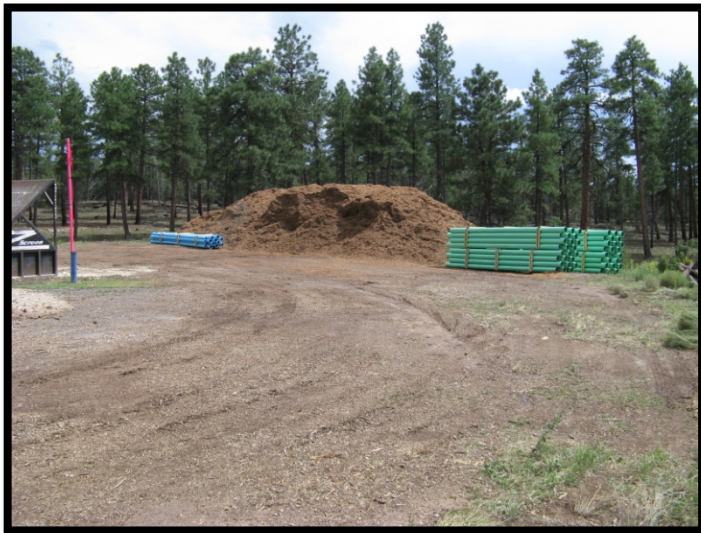
Chip/shred mulch pile staged at a construction site until it was used around the site following project completion.
