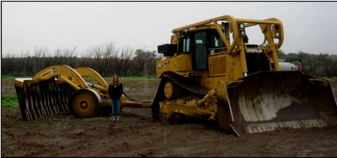
Figure 3.5 Large equipment (Caterpillar D-8) incorporating a deep root rake, Bosque del Apache National Wildlife Refuge, NM, 2007.
