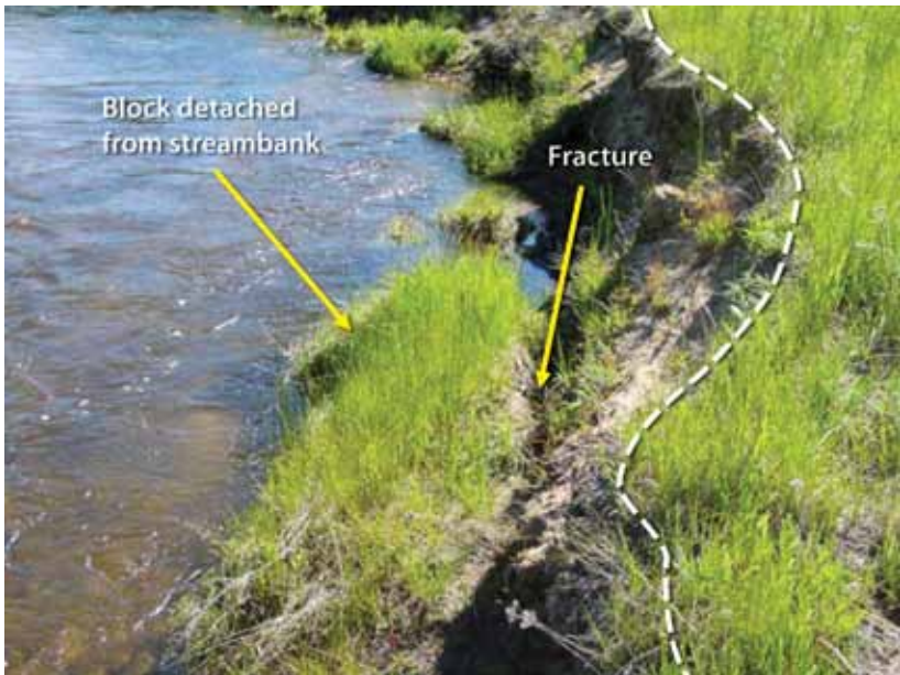
Figure A24. The slump block is detached from the bank wall and there is an obvious fracture between the slump block and the streambank wall. The greenline is located on the streambank as shown.
