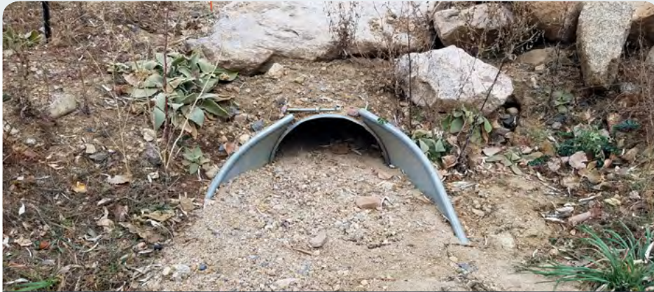
Clogged culverts can cause flood damage to upstream and downstream properties.
