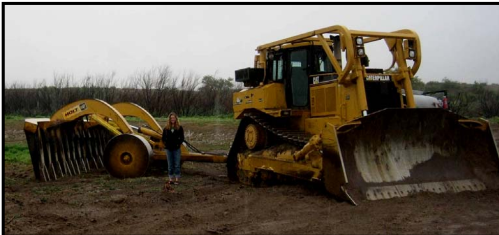
Figure 5: Large equipment (Caterpillar D-8) incorporating a deep root rake, Bosque del Apache National Wildlife Refuge, NM. 2007
