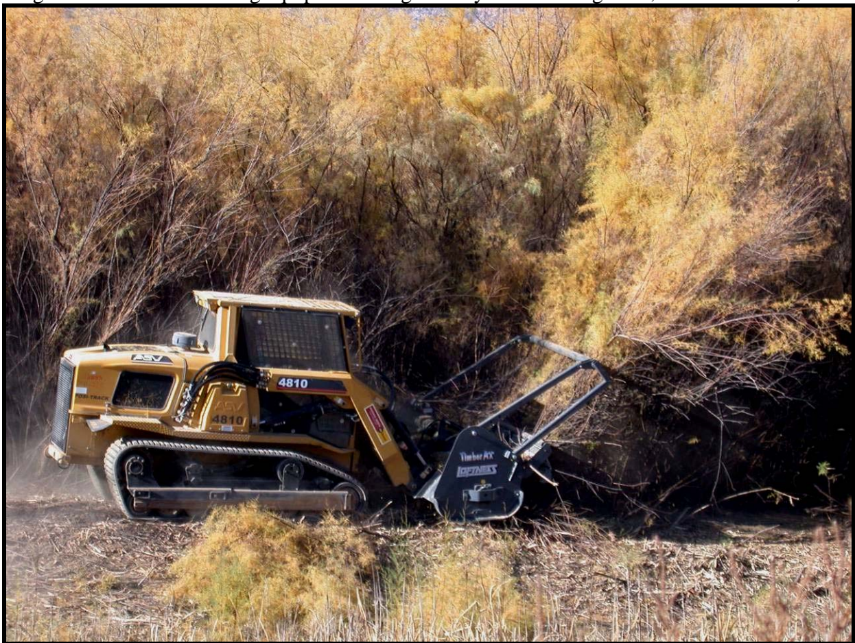
Figure 7: 100 HP mulching equipment using a rotary drum cutting head, Grand Junction, CO.
