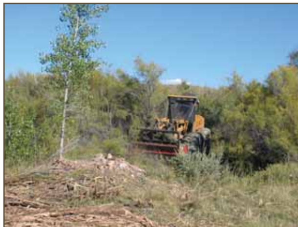
FIGURE 7. A site preparation tractor equipped with a forestry mulching head clears tamarisk on the upper Arkansas. In the foreground is a mulched tamarisk next to a cottonwood. This management tool can be highly selective, but is expensive. When mulching live trees re-sprouts should be treated the following year. (Photo by Stephanie Gieck)
